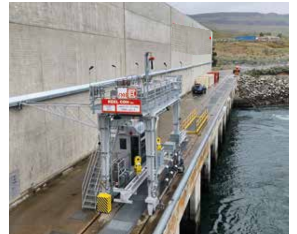
Downstream gantry crane
